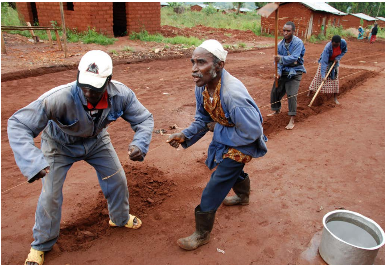
Local volunteers work together to build a road for their community in Burundi (UNDP Burundi/Aude Rossignol, 2013).
